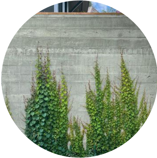
Slot garden to north western footpath to allow climbing plants to grow up the wall and soften presence from street
