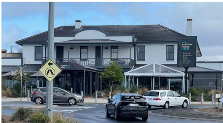
Fig 13: The c1980s parapet, balcony, free-standing pole signage and street pavilions will be removed and are not of heritage significance. The existing windows and doors on the upper level of the hotel facing Ewing Blyth Drive have been altered in the central section associated with the balcony. (H Lardner 22/04/2025)
