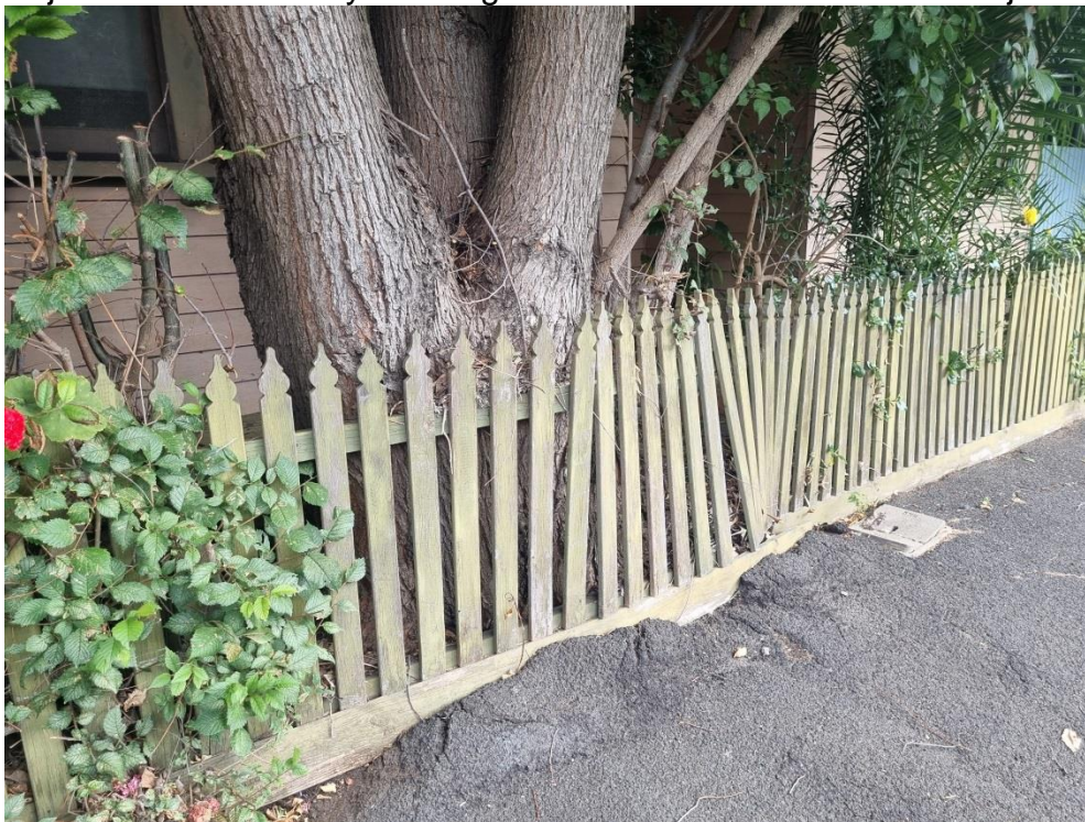
Existing tree to be removed, structural damage to immediate area and potential at risk damage to the building. Distance to the building is less than 1 M.
