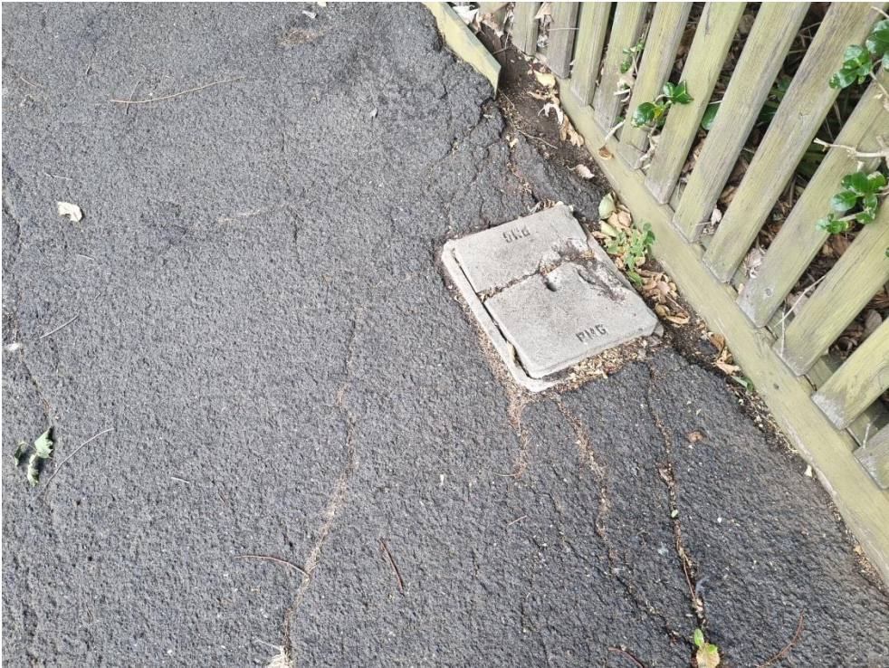
Damaged telecommunications pit.
