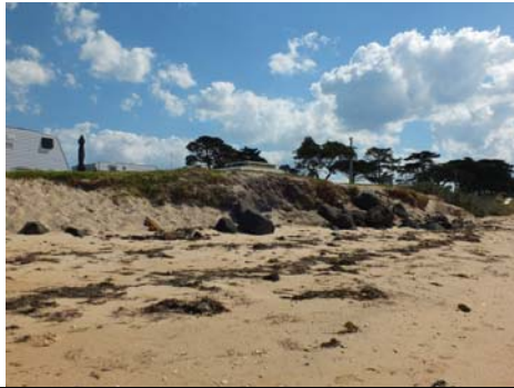
Photo 3.13: Rock revetment in disrepair at Batman Park Foreshore outcrop.
