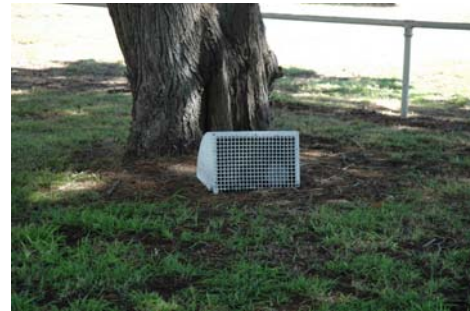
Photo 3.54: Detail of one of the floodlights.
