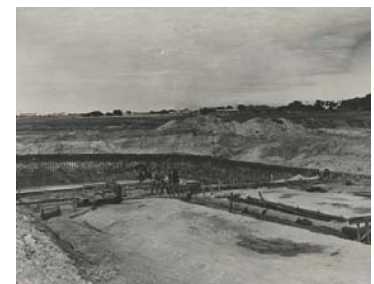
Figure 9.06: McClelland Swimming Pool under construction, c.1962. Source: Geelong Heritage Centre Image Library, image 1263-08-395.
