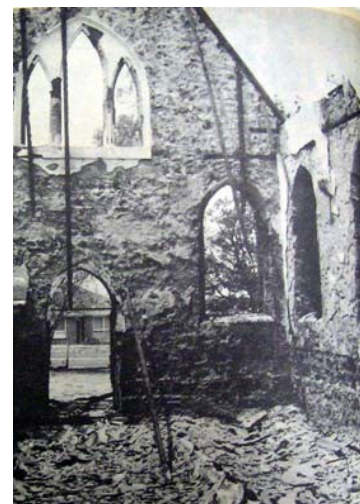
Figure 1.13: Interior of burnt out Holy Trinity Church, 1969. Source: Geelong News , 15 January 1969.
