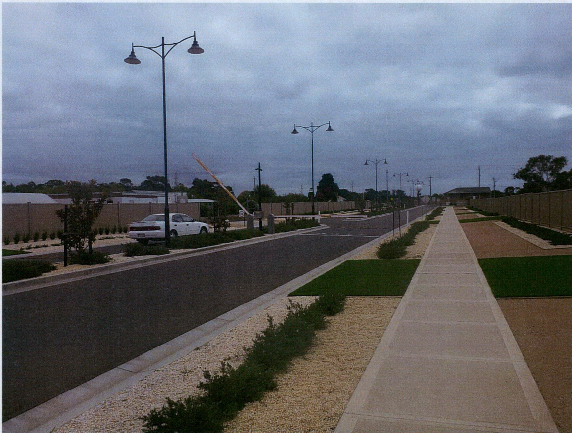
Photo 5: Entry Road with Aged Care Facility construction entry road on right and Flower Farm on left
