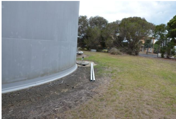
Plate 4: Showing the disturbance surrounding the water tank.
