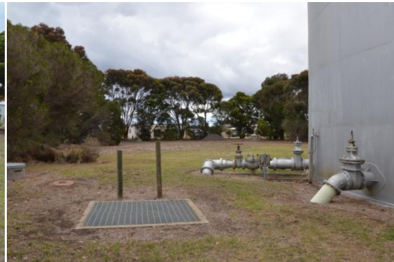
Plate 5: Showing pipe infrastructure.
