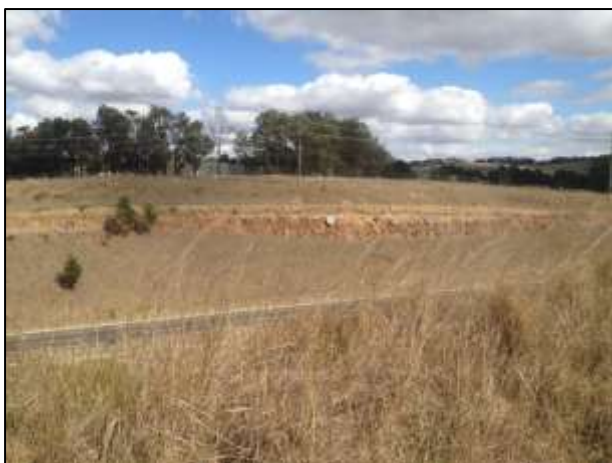
Plate 7: Cutting through the ridge crest for the Ring Road, south west of the study area, looking west
