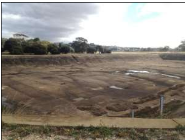
Plate 9: Concrete storage basin covering the eastern half of the study area, looking north west
