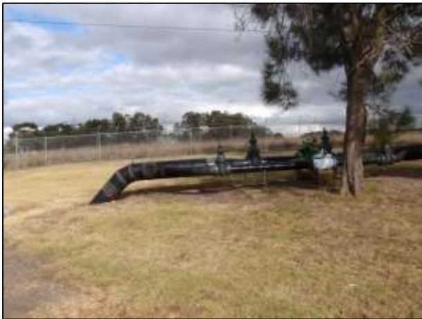
Plate 19: Above ground mains valve near entrance gate on Thornhill Road, looking south west
