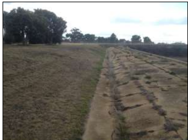
Plate 10: Concrete apron and drain along the western side of the basin, with modified grassed area to the west, looking north
