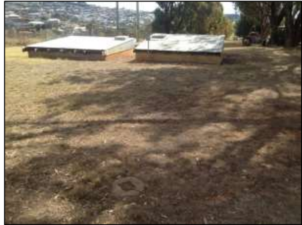
Plate 18: Valve covers for the mains pipelines along the western boundary of the study area, looking north towards the creek slope
