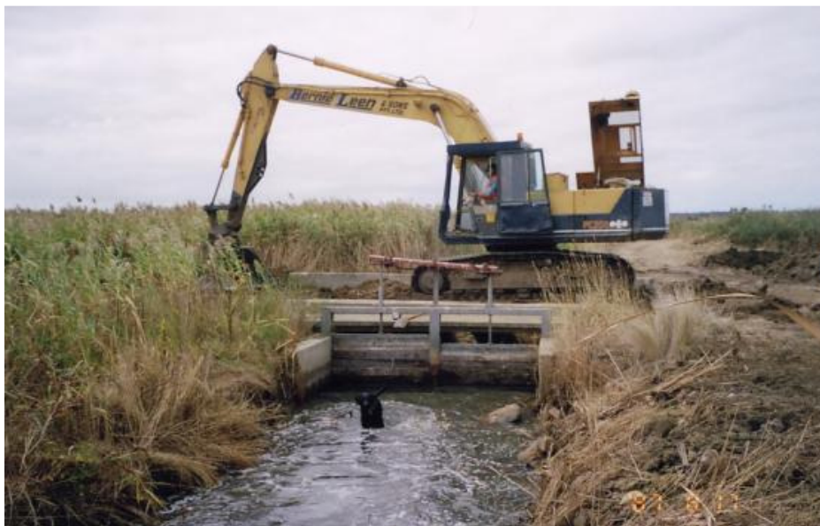
Figure 2-3 Reedy Lake Outlet Regulator Structure
