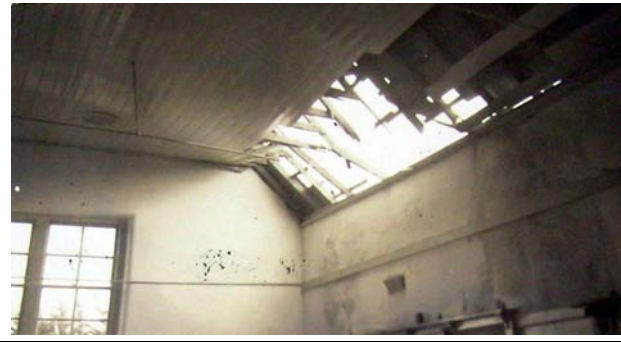
Figure 7: Interior, Ceres State School showing roof damage, 6 December 1948. Source: VPRS 10516/P3 Unit 7 Public Record Office Victoria.
