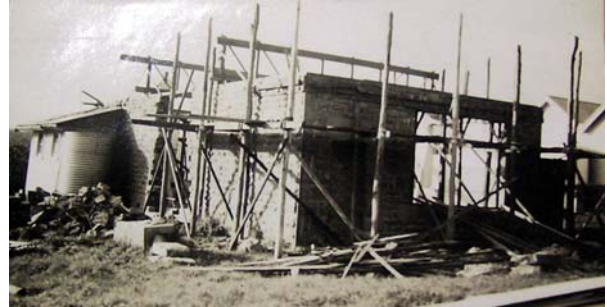
Figure 12: Ceres School under construction (south & west elevations), 15 Sept 1950. Source: VPRS 10516/P3 Unit 7 Public Record Office Victoria.
