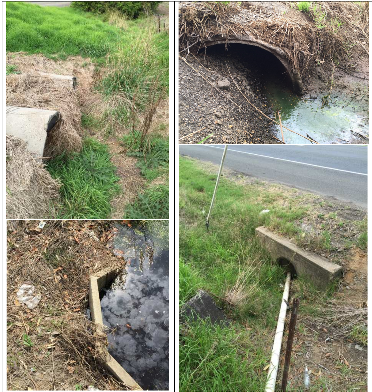
Figure 6-3: Field inspection photographs – culvert condition
