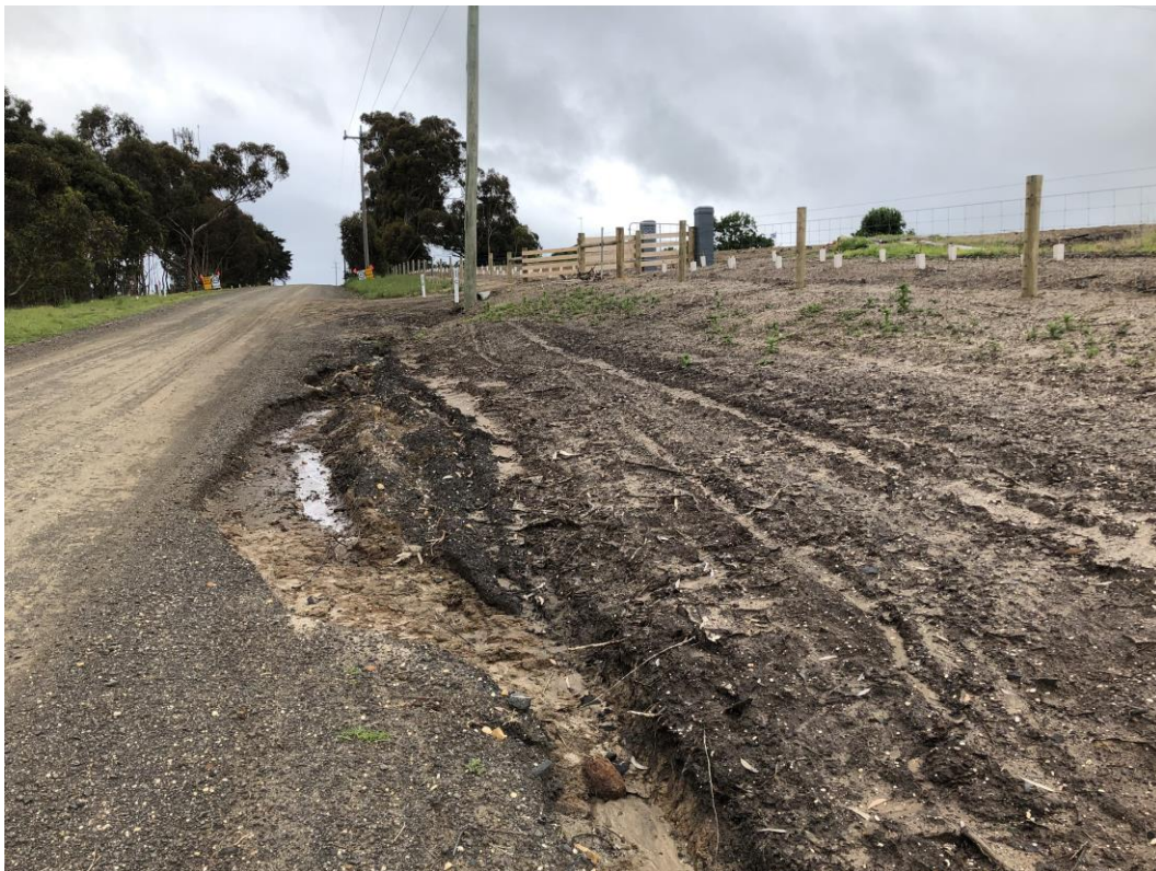
Photo 11 – View north on Mollers Lane (east side) from north of Tributary 1 crossing. Evidence of erosion and from recent rain
