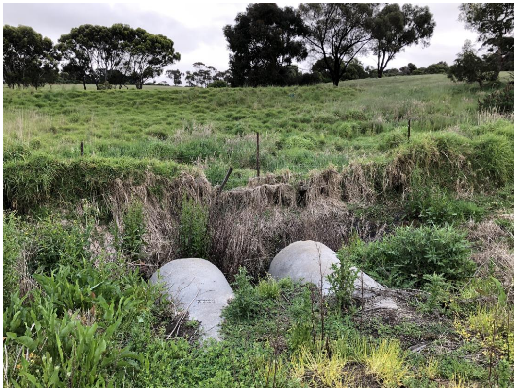
Photo 8 – View west from Mollers Lane at upstream side of Tributary 2 crossing. Culverts in foreground and farm dam background
