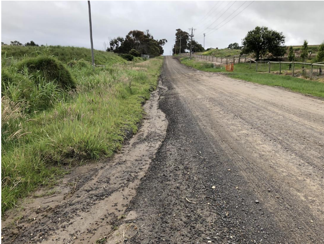
Photo 10 – View north on Mollers Lane from Tributary 1 crossing. Evidence of erosion and sediment deposition from recent rain
