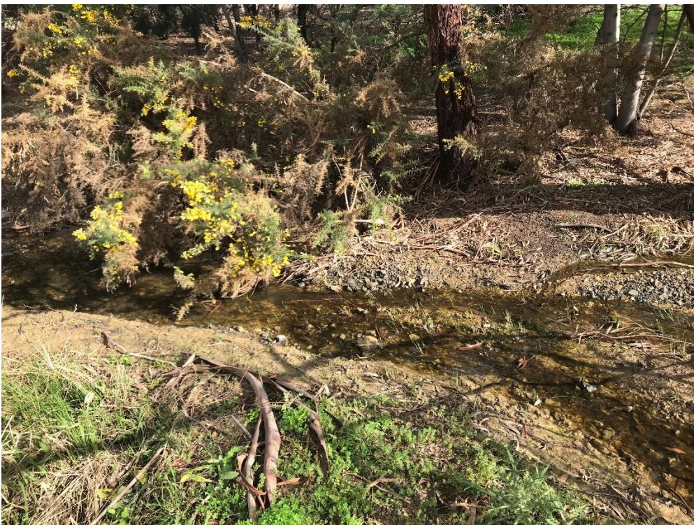
Existing waterway downstream of railway culvert full of sediment.
