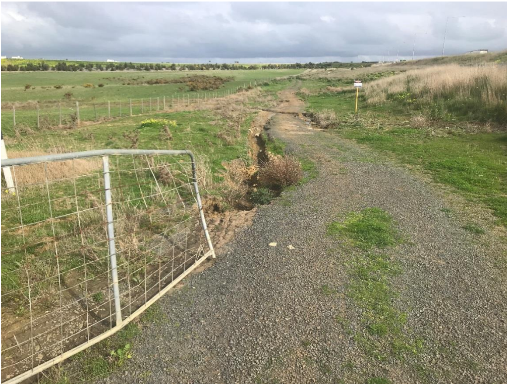
Erosion within the upstream road reserve (outlet from VicRoads culvert from the west)
