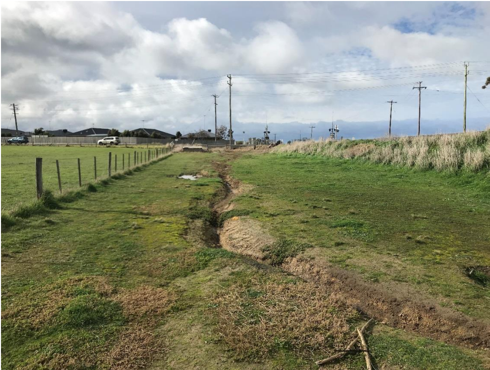
Erosion within the upstream side of the rail reserve (from the east and Ghazeepore rd)
