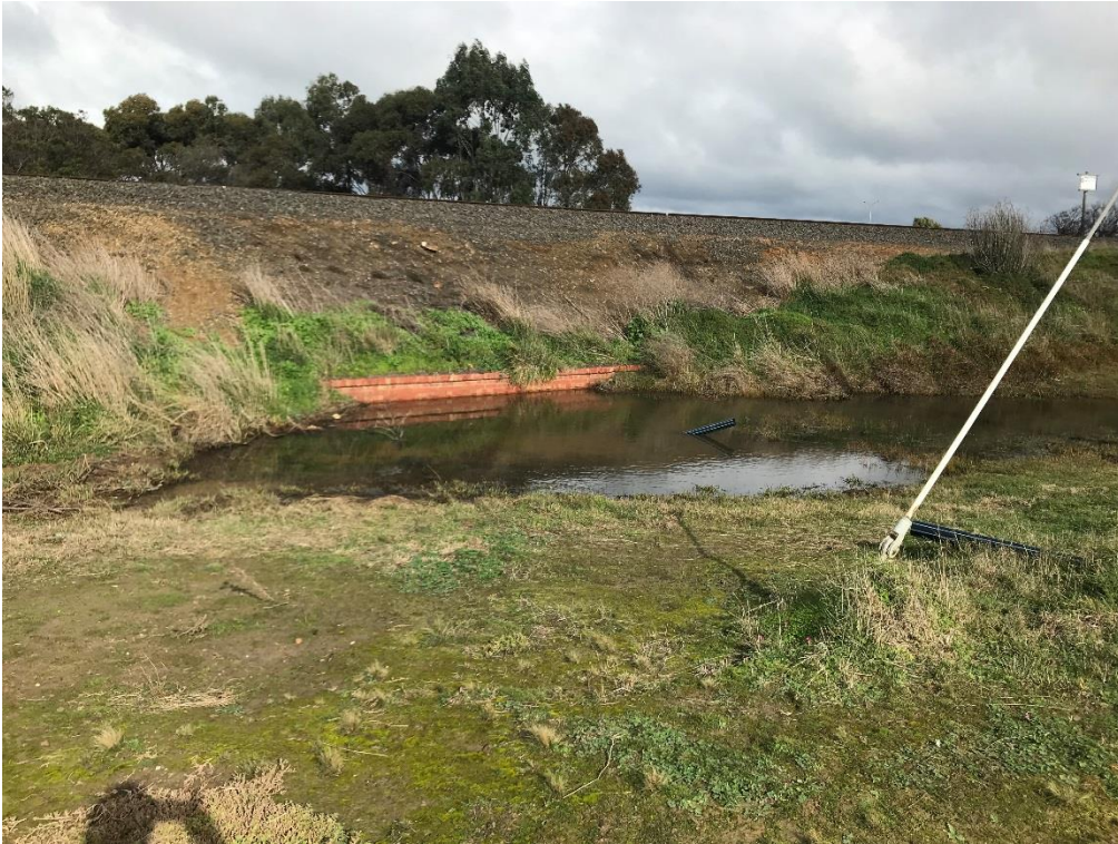
Existing Warrnambool - Geelong railway Culvert submerged (upstream)
