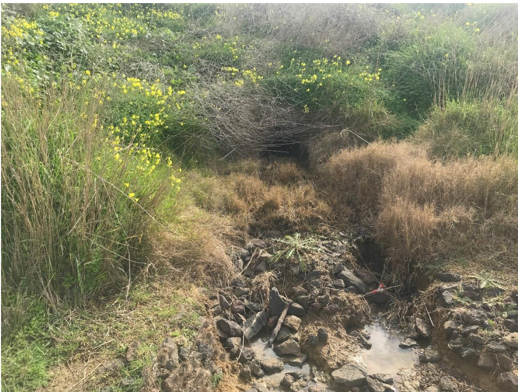
Erosion within the upstream road reserve (outlet from VicRoads culvert from the west)
