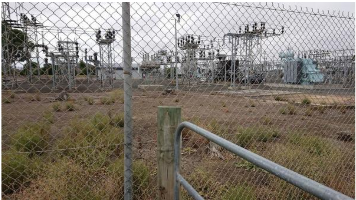
Photograph 8 Substation in NE of site.
