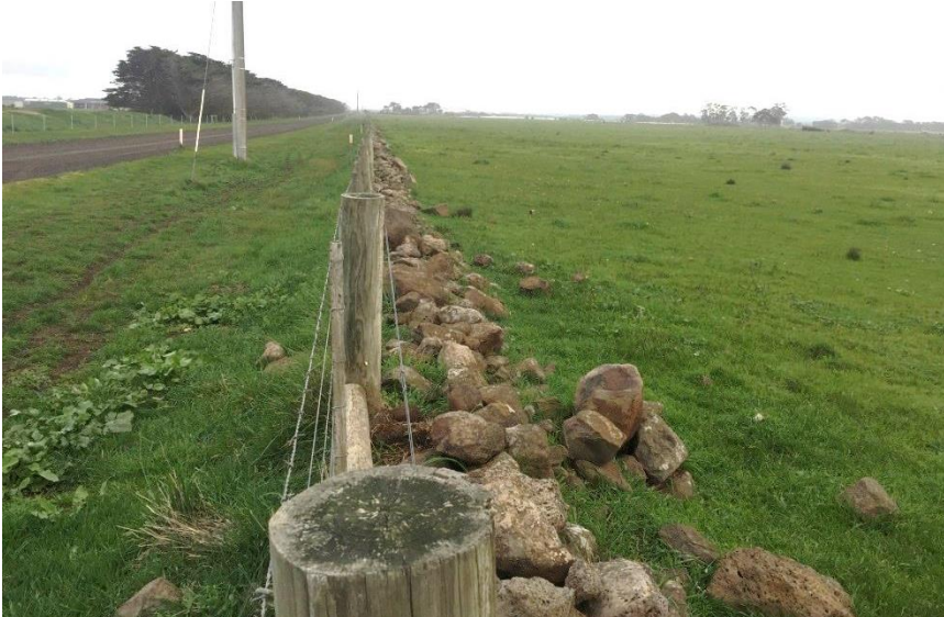
Plate 5: A section of dry stone wall on the western side of Evans Road
