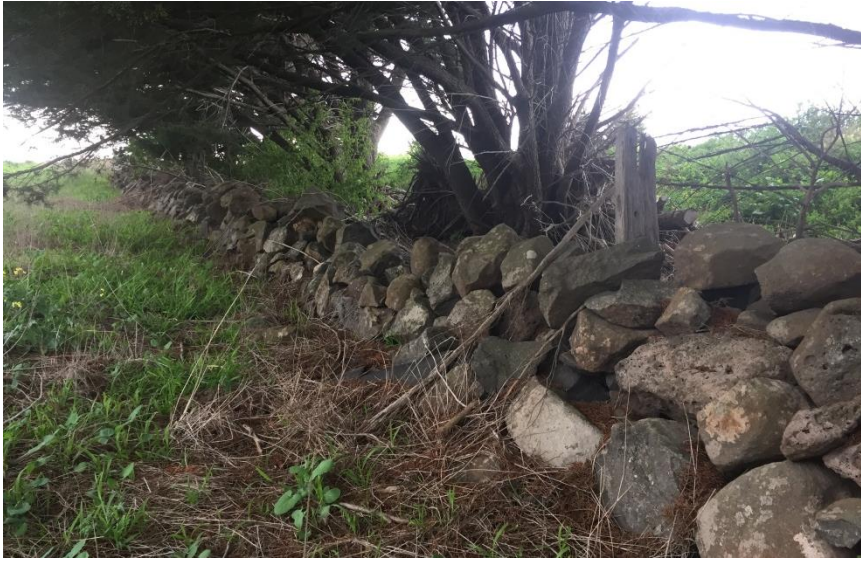
Plate 4: A remnant section of dry stone wall on the eastern side of Anakie Road
