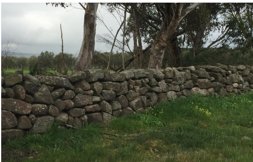
Plate 2: A section of all-stone dry stone wall on the northern side of Elcho Road
