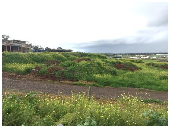
Plate 10: Extensive cut and fill on the escarpment slope for residential developments, looking north
