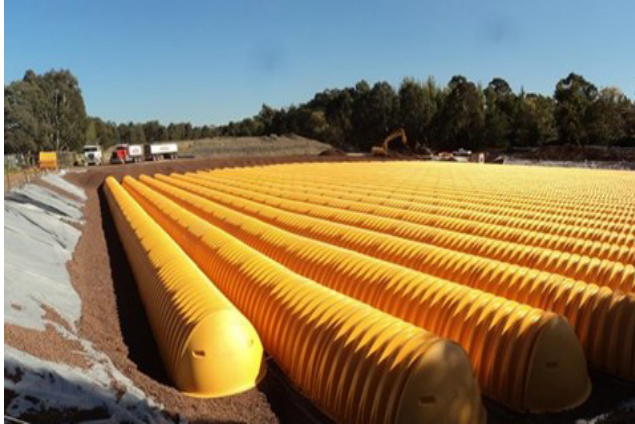
CONSTRUCTION OF ONE SECTION OF THE BANYULE STORMWATER HARVESTING PROJECT (IMAGE: WWW.202020VISION.COM.AU)
