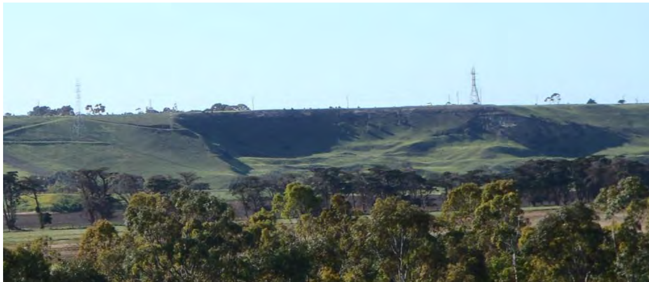
Photo 7 : View of the historical landslide at the downstream end of the Moorabool Deviation Channel
