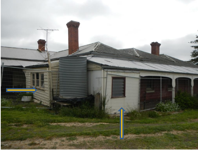
Figure 4 The timber and cement sheet additions to the south-east corner of the east verandah.
