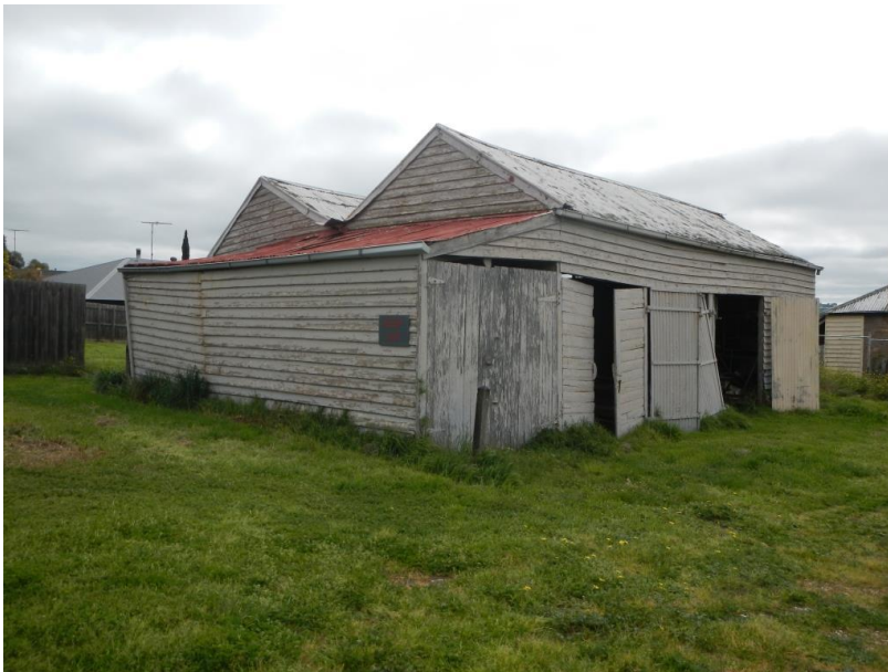
Figure 5 The east and south elevations of the detached double gabled timber weatherboard outbuilding.
