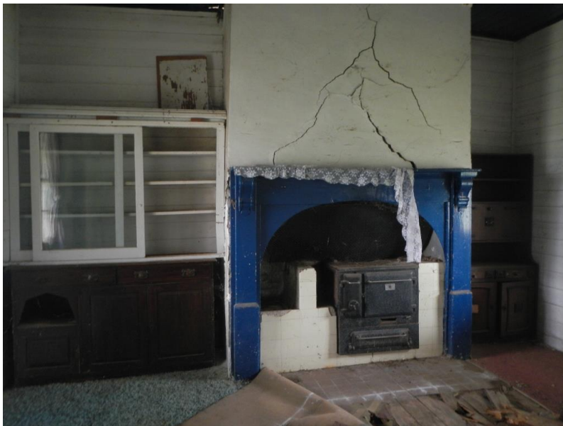
Figure 13 The kitchen is highly intact and retains its timber-boarded ceiling, wide lining boards to the walls, chimney breast, hobs and solid fuel stove and old cupboards. The dilapidation is repairable. Most probably the chimney would need to be taken down and reconstructed and a new floor installed.
