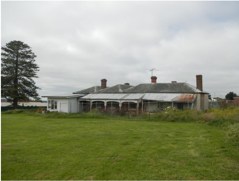
Figure 12 The west elevation of the homestead and the kitchen wing. While is poor but repairable condition, it is mostly intact. The well is about the location of the join in the verandahs.
