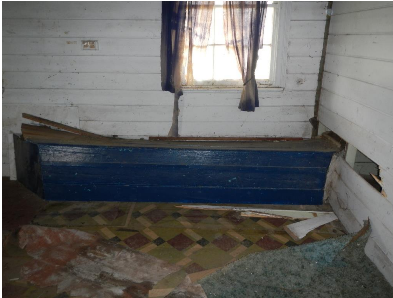
Figure 14 The kitchen is highly intact and is probably unique in Waurn Ponds and probably rare in Victoria. The indoor part of the well is in the blue "box". Note the wide lining boards.
