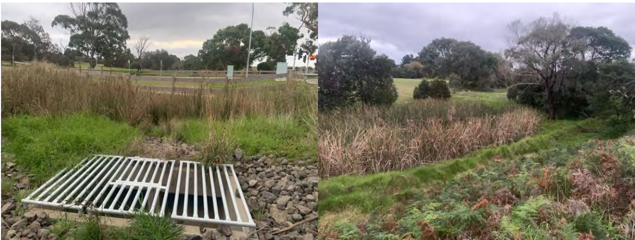
FIGURE 7-1 LEFT: GRATED PIT UPSTREAM OF TIVOLI DRIVE & RIGHT: DAM LOCATED UPSTREAM OF THE CULVERT UNDER RAIL TRAIL EMBANKMENT
