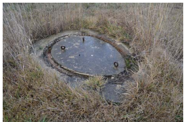
Ovoid concrete plate remnant.
