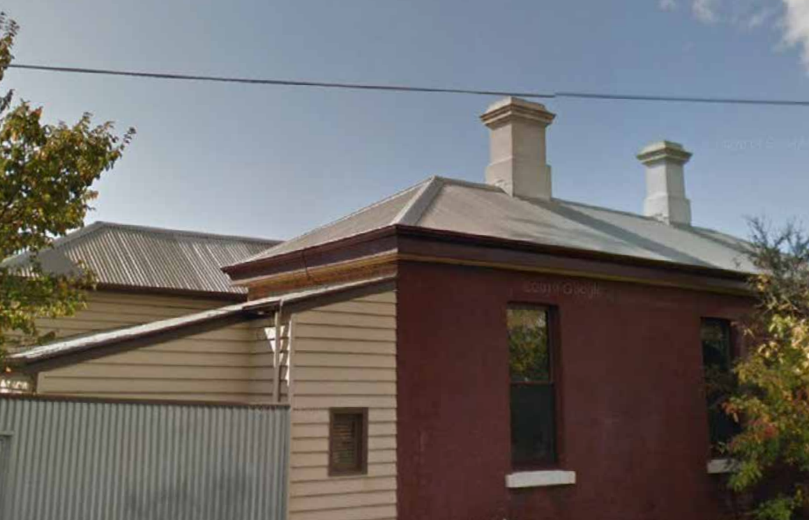
Figure 3. View of 'Kardinia Villa' (east elevation) from Moorabool Street. Source: David Scott, City of Greater Geelong, 2022.
