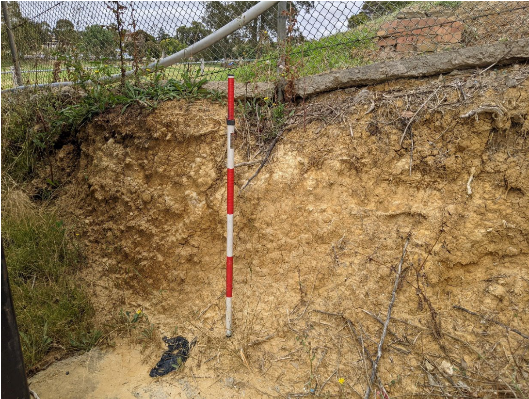
Figure 41: Exposed embankment cut, facing west (C. Hawker, 22 February 2022)
