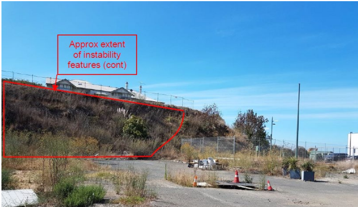
Figure 25: Northern batter, facing north east showing instability as marked in geotechnical study (Douglas Partners 2019)
