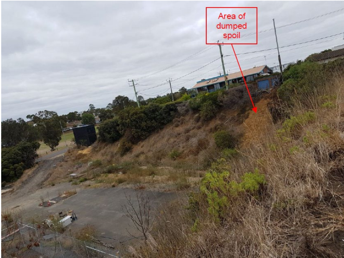
Figure 23: Current condition of activity area, facing south-west, showing western batter (Douglas Partners 2019)
