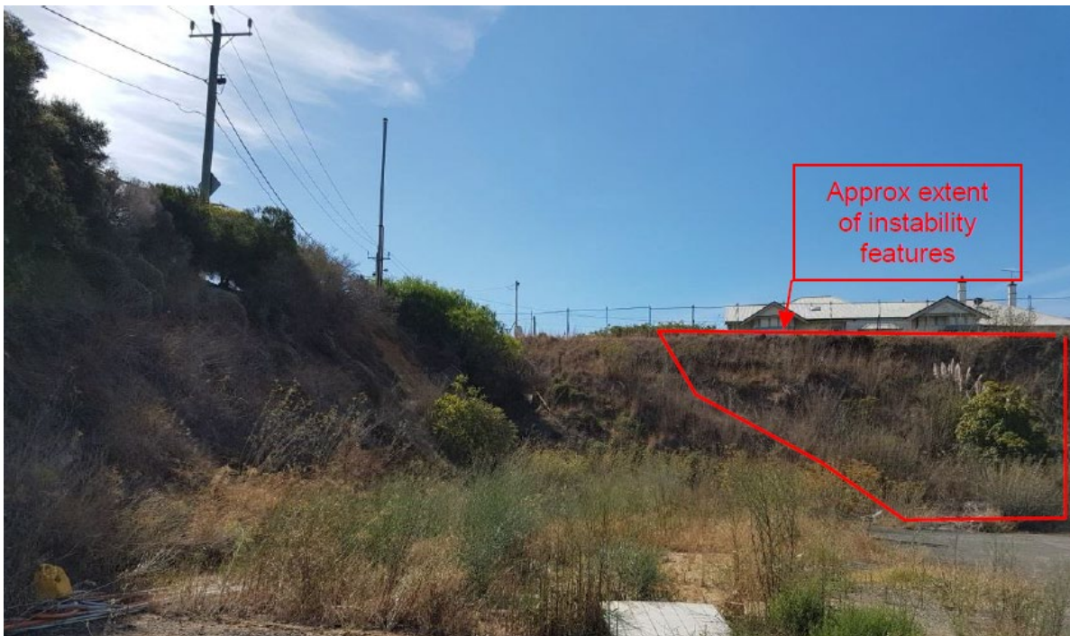
Figure 24: Northern batter, facing north showing instability as marked in geotechnical study (Douglas Partners 2019)
