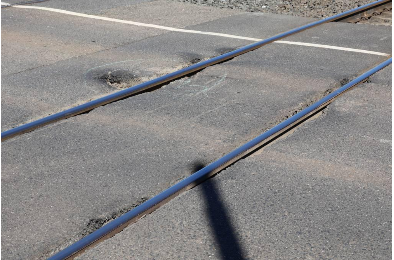
Figure 6 Deep Holes in ARTC track panel
