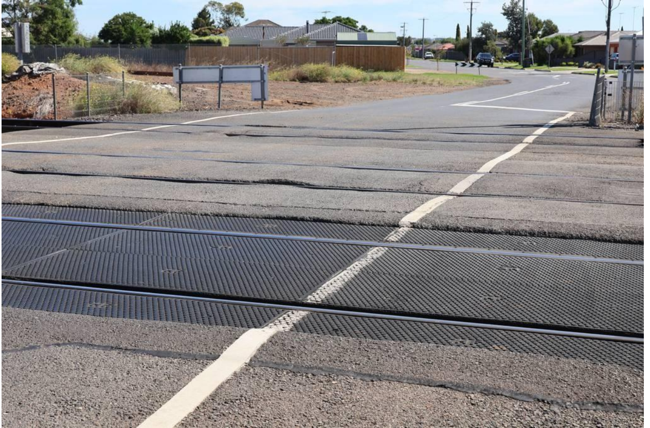
Figure 5 Road Condition Eastbound
