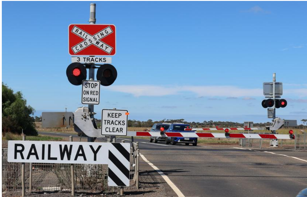
Figure 9 Boom barrier controls on eastern crossing approach
