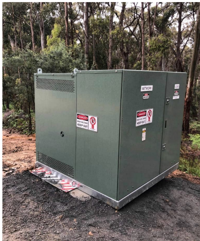
Figure 21: 1000kVA REFCL isolating transformer, physical size is similar to a kiosk substation
