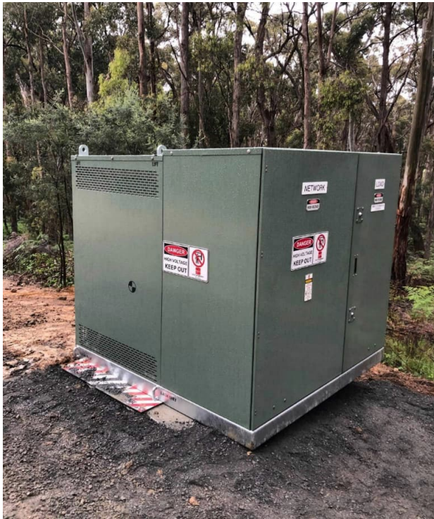
Figure 2 - 1000kVA REFCL isolating transformer, physical size is similar to a kiosk substation
