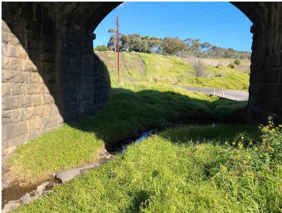
Photo 12 Existing underpass of Cowies Creek at Bluestone Bridge Road. Looking approximately south
