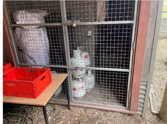
Photo 2: LPG gas tanks stored onsite.
