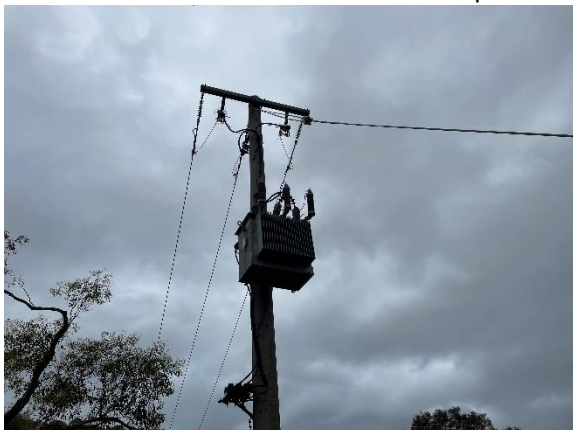
Photo 5: Transformer on power pole within site boundary.
