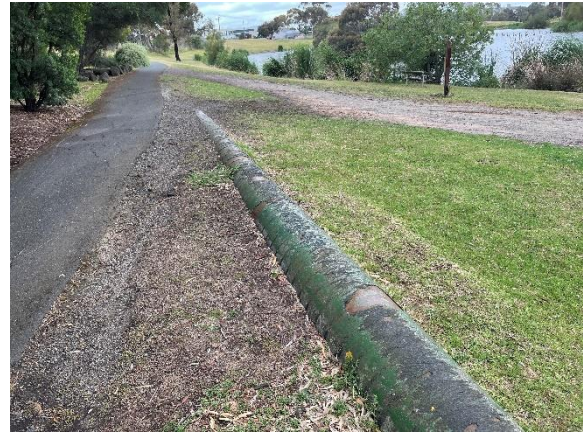
Photo 8: Water main pipe with suspected asbestos-containing coating.
