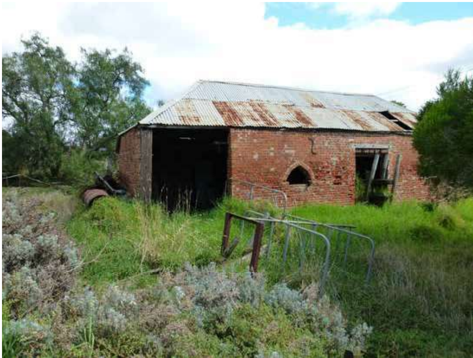
Figure 4: Stables, east elevation showing later opening, temporary door barrier, fencing and site rubble. Source: David Scott, City of Greater Geelong, 2022
