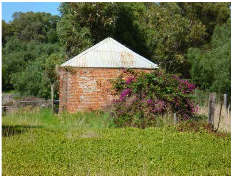
Figure 5: Stables, north elevation showing wall subsidence, and penetration of external walls by plants. Source: David Scott, City of Greater Geelong, 2022.
