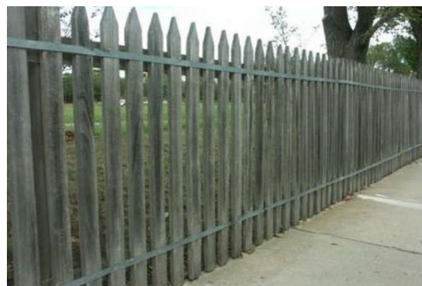
Figure 69 Unpainted timber picket fence with hoop iron used to reinforce the pickets
