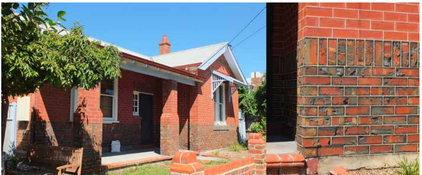
Figure 11 Bungalow, Newtown, 1920s. Bungalow featuring distinctive brickwork construction enhanced by tuckpointing repairs.
