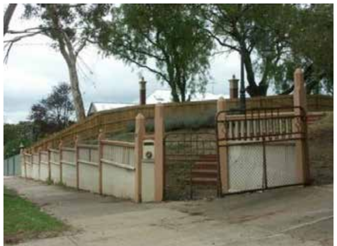
Figure 78 Detail of Federation era ripple iron and timber fretwork fence, with scrolled metal and wire vehicular and pedestrian gates.
