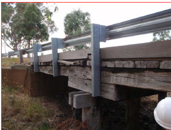
Poor – (Lees Road North)
